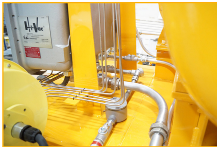
CONDUIT ISOLATED WIRING
